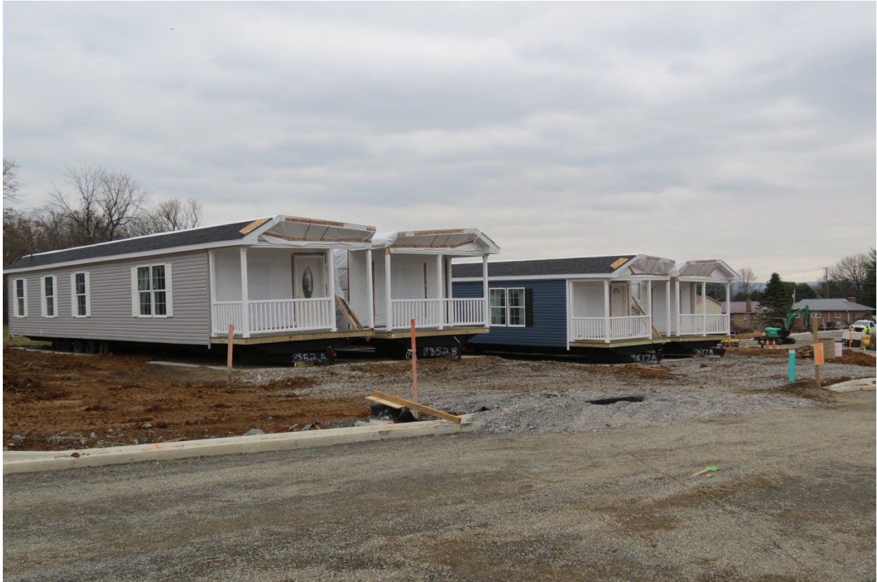
Two of the first homes in Kilpatrick Woods shortly after being sited, awaiting the raising of their roofs. Since CrossMod™ homes have higher roof pitches than traditional manufactured homes, builders often use hinged roof systems which allow the roof to be raised only after being transported and installed on site.
